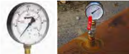
Fig. 1.5.83 Typical pressure gauge and transmitter installation
