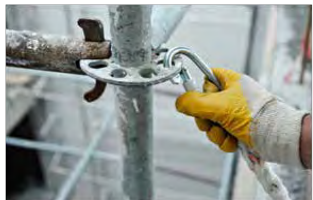
Fig 2.3.2. Wrong Anchoring / Clamping
