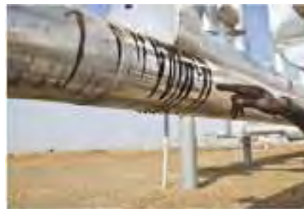
Fig. 4.3.31 Pipeline leak due to 3rd party attack
