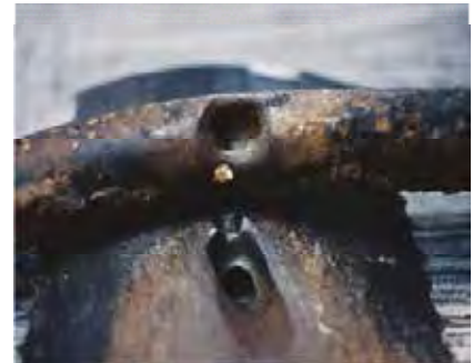
Fig. 4.3.35 Pipeline explosion due to corrosion
