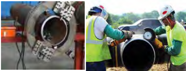
Fig. 1.7.9 Beveling and cutting equipments
