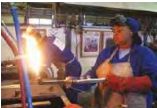
Fig. 4.3.17 Example of unsafe act
