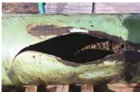
Fig. 4.3.30 Pipeline rupture due to fatigue crack.
