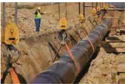
Fig. 4.3.19 Pipe lowering in unsafe condition (standing very near to trench edge)
