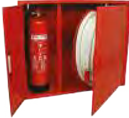
Fig. 4.2.11 Firefighting hose reel
