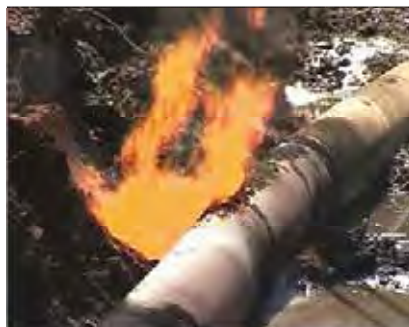
Fig. 4.3.34 Pipeline explosion due to rupture
