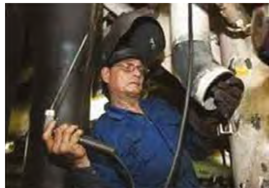
Fig. 4.3.18 Example of Unsafe acts and unsafe condition
