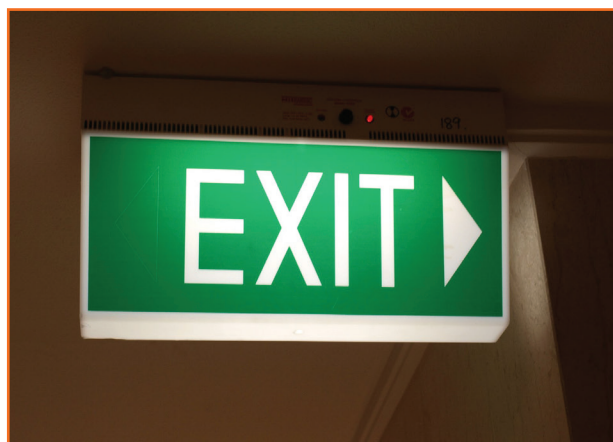
Fig: 2.1.7 Exit Sign
