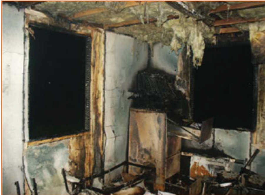
Fig: 3.2.5 Gathering information at site after accident
