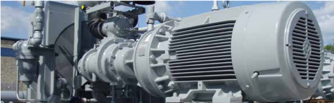
Figure 2.4.5: Sample of a rotating equipment used in the oil and gas industry
