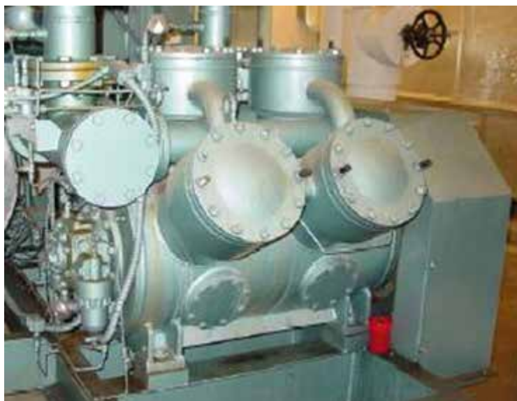
Figure 2.1.8: A six-cylinder Reciprocating Compressor
