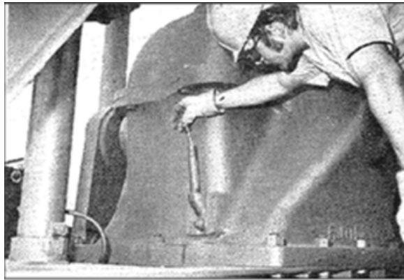
Figure 2.3.6: Worker inspecting the gearbox at the work site
