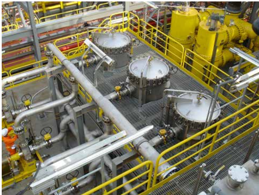
Figure 2.4.3: Sulphate Removal Package at the site of work
