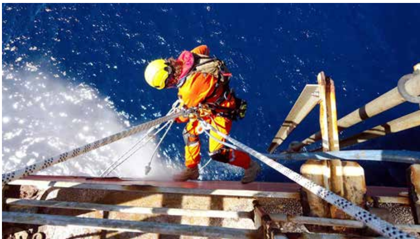
Picture 2.2.2: Fall Protection System
