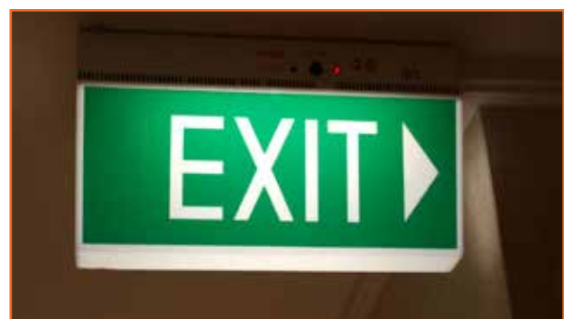
Fig: 5.1.8 Fire Safety Sign
