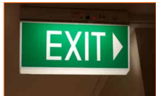
Fig: 2.1.32 Photo Luminescent Sign
