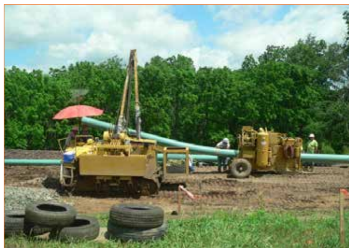
Fig: 2.1.13 Contouring or bending pipe to fit the contours of the landscape
